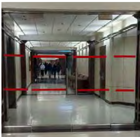
Contributed by Josh Archilla, Staff Photographer New doors are in place at what will be the new entrance to the Performing Arts wing.
