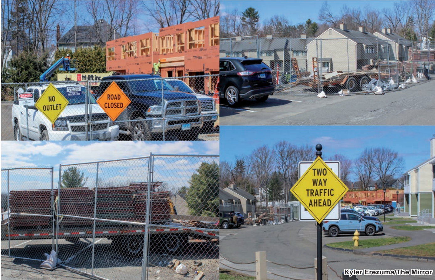
Construction in the Townhouse area began in the fall semester. Students were notified on March 10 that progress with the construction of two new Townhouse blocks would cause traffic changes for the rest of the spring semester.
